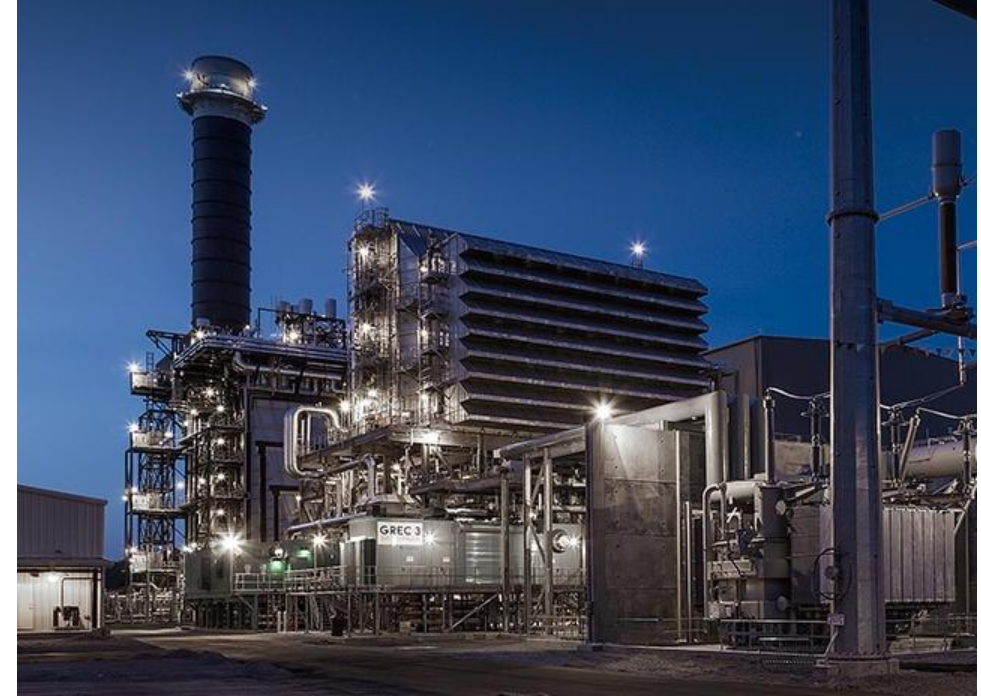
Gas Turbine Combined Cycle Mitsubishi 501J Grand River Dam Authority
