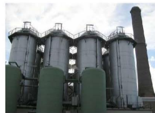
Steam Accumulators: 1929 Charlottenberg Power Station, Berlin
