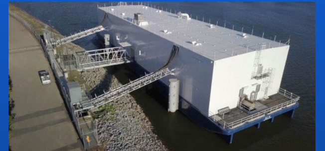
Vessel data center Commissioning for the world's first zero-water consumption data center
